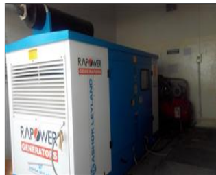
External photo(s) of the production unit(s) Genset.jpg
